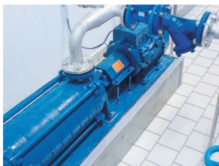
▲ Ecological energy generation with ANDRITZ Ritz pump turbines at a German water supply network
